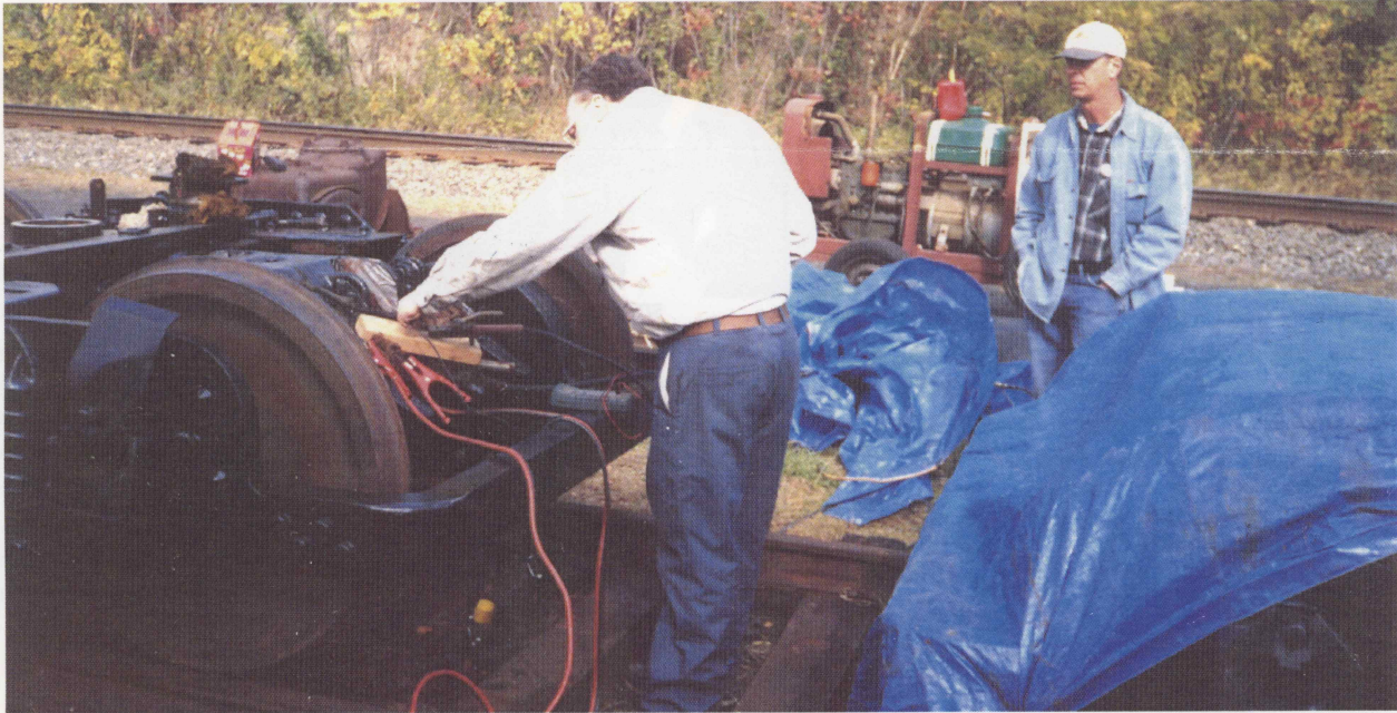
Carl Hosler oversees the testing of one of the trucks for car 2651. The electric motors performed flawlessly and the truck moved slowly along the section of track in front of the building where our car is stored. Plans for this fall call for removing the caboose trucks now under the car and replacing them with the motor trucks. Photo by Tony Hall
