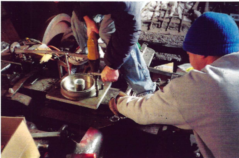
Jim Tomczyk and Rob Hooper are shown matching up holes in new center bearing with those in power truck beam. Some re-drilling would be required to fit bolts.
