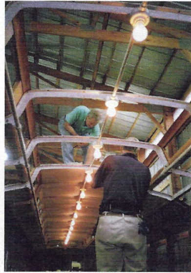
(Above) Bob Hooper fiddles on the roof as Hank “The Plank” Kaminski holds the nuts ensuring progress on installing the new center roof panels on ex-PSR car 2651.
