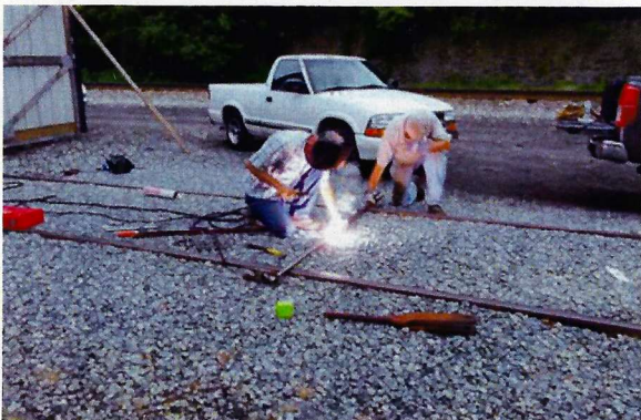
Bob assists Glenn in the welding of the two brake link sections. Tony Hall photo, 6 August 2011.
