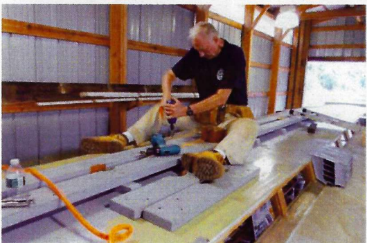
With drill in hand, Hank prepares for the bolting of the west-end walk boards. Tony Hall photo, 20 August 2011.
