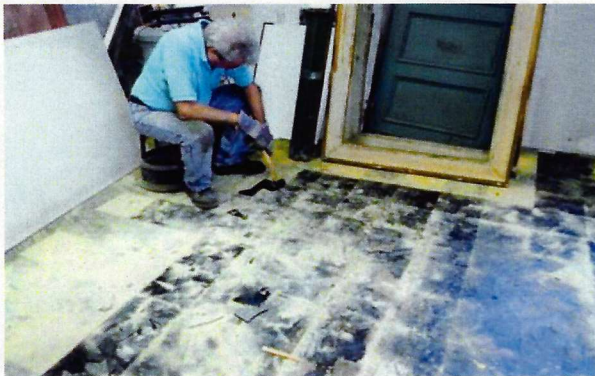
Working in un-air conditioned discomfort, Bob painstakingly removes floor tiles applied in recent years by a prior commercial tenant in the station. Tony Hall photos, 10 September 2011.
