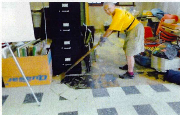
In additional views, Ken Miller is, assisted by a shadowy second-story man, removes the now unneeded ducts and conduits, while Ann Miller and Tony help with removal of floor tiles. Bob Hooper photo, 10 September 2011.
