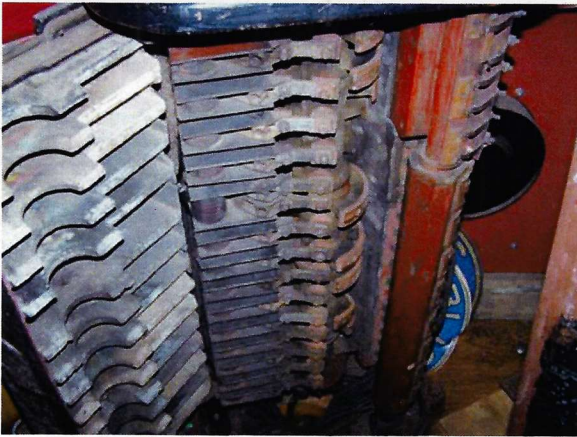
The east controller is dissected, revealing its complex electro-mechanical organs. Tony Hall photo, October 2011.
