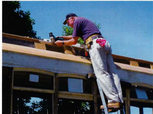
The upper trim molding required some last-minute routing to accommodate the ventilators. Bob Hooper photo, 1 July 2011.
