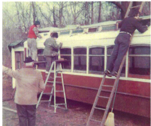
As ladder day trolley saint, Frank climbs to heretofore new and unfamiliar heights in pursuit of a new roof for 2651.
