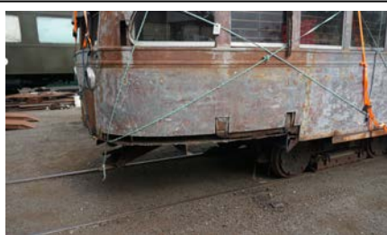
The right rear gets the same treatment to its rusted skin and floor plate.
