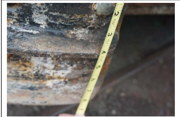
The left quarter of the front anti-climber had been badly damaged in an accident.
