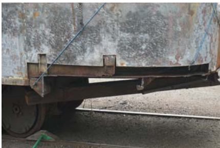
The left rear of the outer body skin has been plasma torched to remove the rusted material at the floor line.
