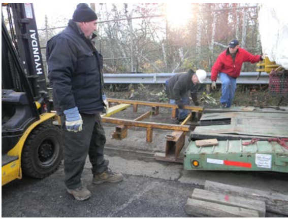
Figure 19: The Ramp rails must be aligned meticulously with both the trailer rails and those of the unloading track.
