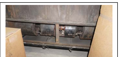
The Newark PCCs are all electric and needed a motor generator to provide 32 volts for the electrical accessories (lights, doors, PA system).
