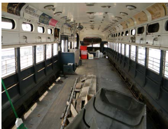
Removal of the seats and heater cover panels has revealed the extent of rust damage and consequently the amount of needed restorative work to come for PCC #13.
