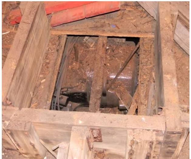
At the bottom of the motor access well, there is, what else? a MOTOR.!
