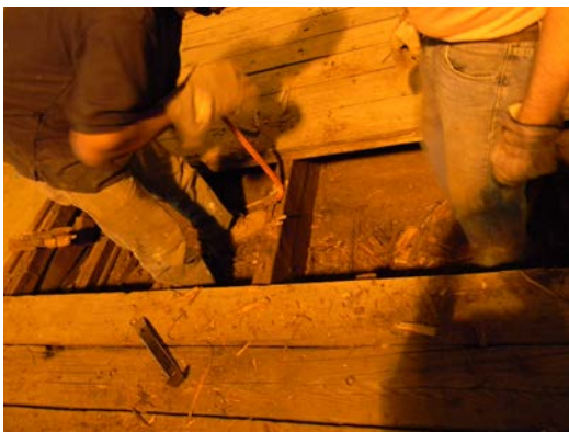
Thirty five feet of heavy decking had to be removed, one plank at a time. After all, we had a dumpster to fill!
