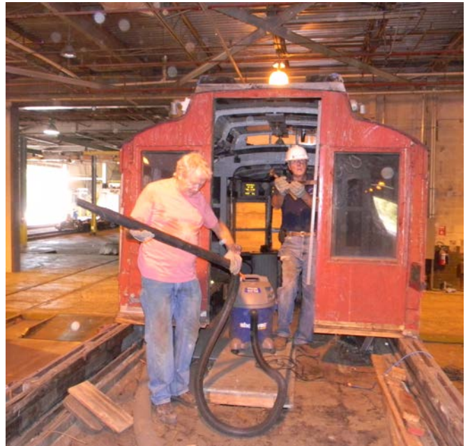
Hoping to see once again the "Deluxe" floor of the 30's, Bob mans the mighty "Shop Vac". But alas the great machine choked on the first snoot-full of wood dust it inhaled. Meanwhile Hank began the dismantling of the cab.
