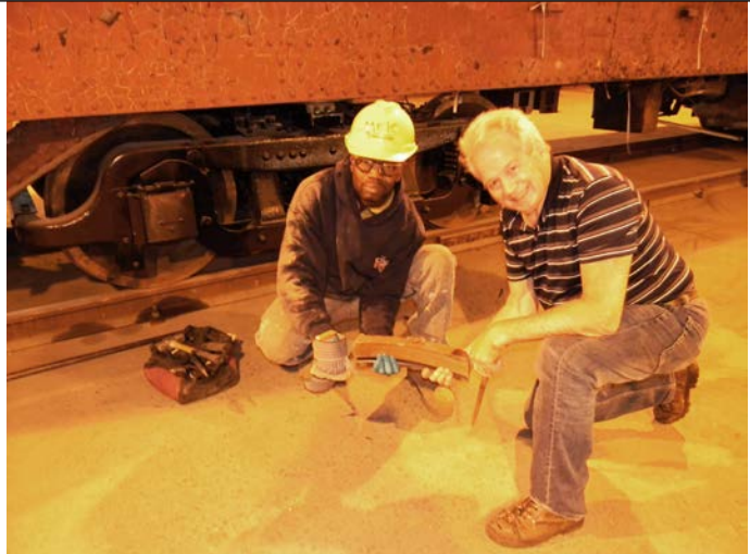
Bob (right) and Carl Pinder (left) of K-S display the brake shoe that was to be installed on the Flat Car.
