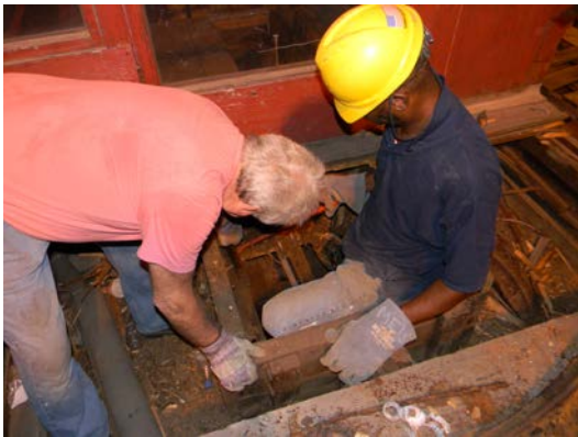
The car's original floor beneath the deck was discovered to be in abominable condition after 100 years of hard use.
