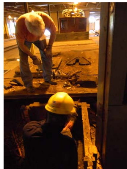
Wells built under the decking gave access to the traction motors below.
