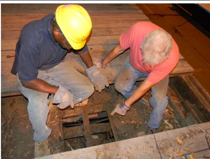
Another deficiency was discovered; namely two missing brake rod connecting pins. Here Bob & Carl discuss the new problem.
