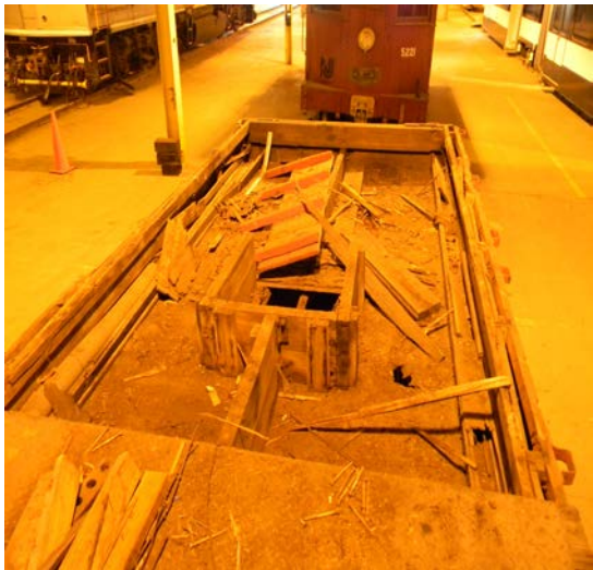
One of the motor access wells, built beneath the deck, is revealed here.
