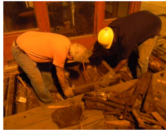
With the help of KS' Carl Pinder(R). Bob begins removing the decking applied by PSR decades ago.
