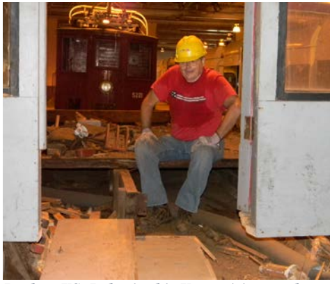
Back at KS, Bob tries his X-ray vision on the old decking of #2683 to determine the extent of the deterioration beneath.
