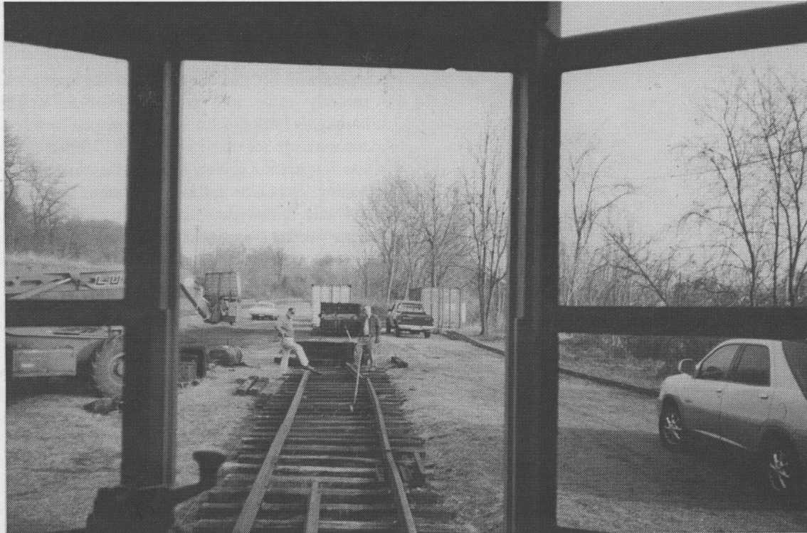
This view through the front windshield of Car 2651 shows the work that was underway on the extension of the track in front of our car barn. The car can now be displayed entirely out in the open. Photo by Tony Hall
