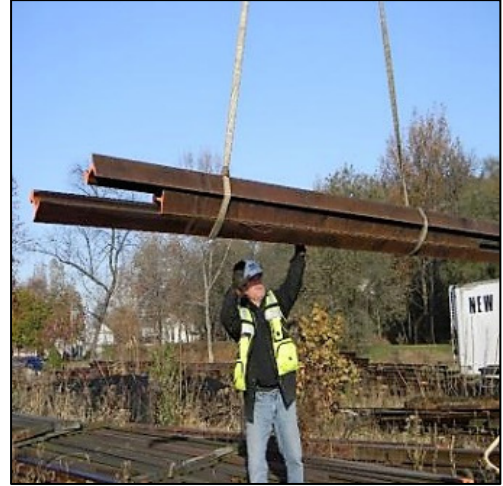
Fig. 8-3. With a little help from on high, Frank levitates the rail and guides it toward the truck.
