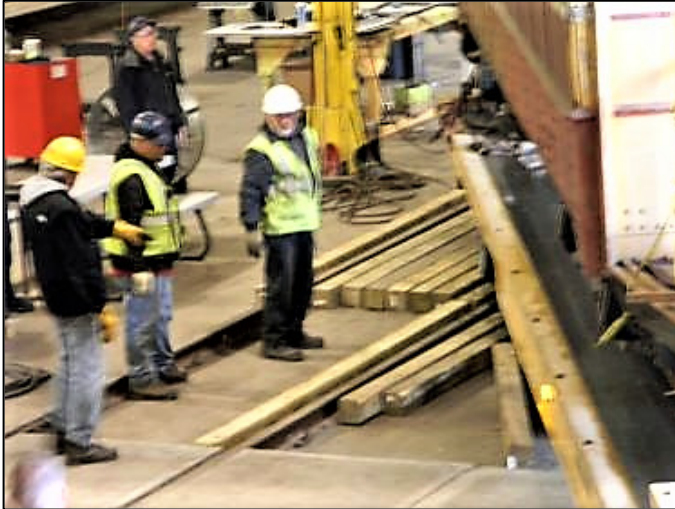
Fig. 17-1. Timbers are placed into the gauge to facilitate the passage of rubber-tired truck wheels over the track
