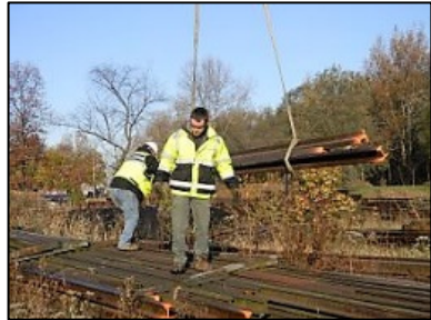
Fig. 8-2. Frank Dunn (Excel Plumbing) and Justin Graupe (City Erectors) select the rail for lifting. Photo: Bob Hooper DSCN3952
