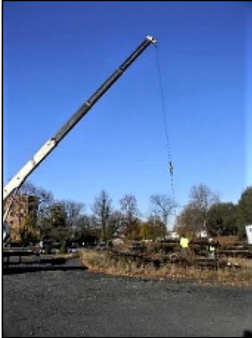
Fig. 8-1 Reach for the sky! A crane was brought in to load rails for transport.
