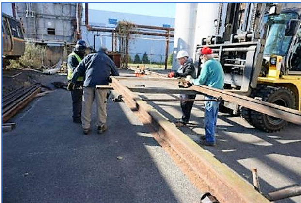
Fig. 9-3. A forklift, operated by a skilled K-S staffer, makes handling hundreds of pounds of steel seem easy. It was not.
