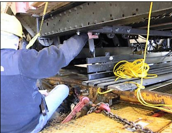
Fig. 15-4. Bob Hooper wrestles with the safety gate. DSCN4048
