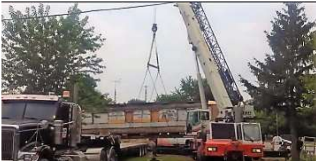
Fig. 10.4 Demolishing the house that contained Car 351. A high price to pay, but WHAT A REWARD! (V7)
