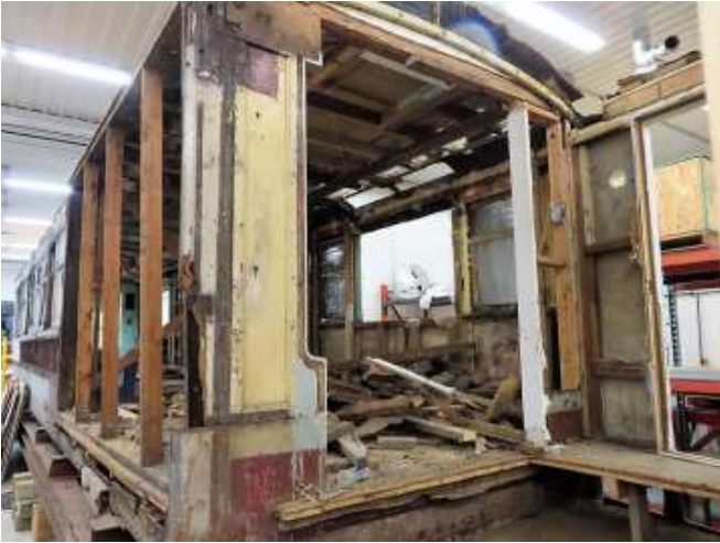
Fig. 12.1 The damage inflicted by the house builders 80 years ago is immediately evident. (Keigher Collection Pt2-4)
