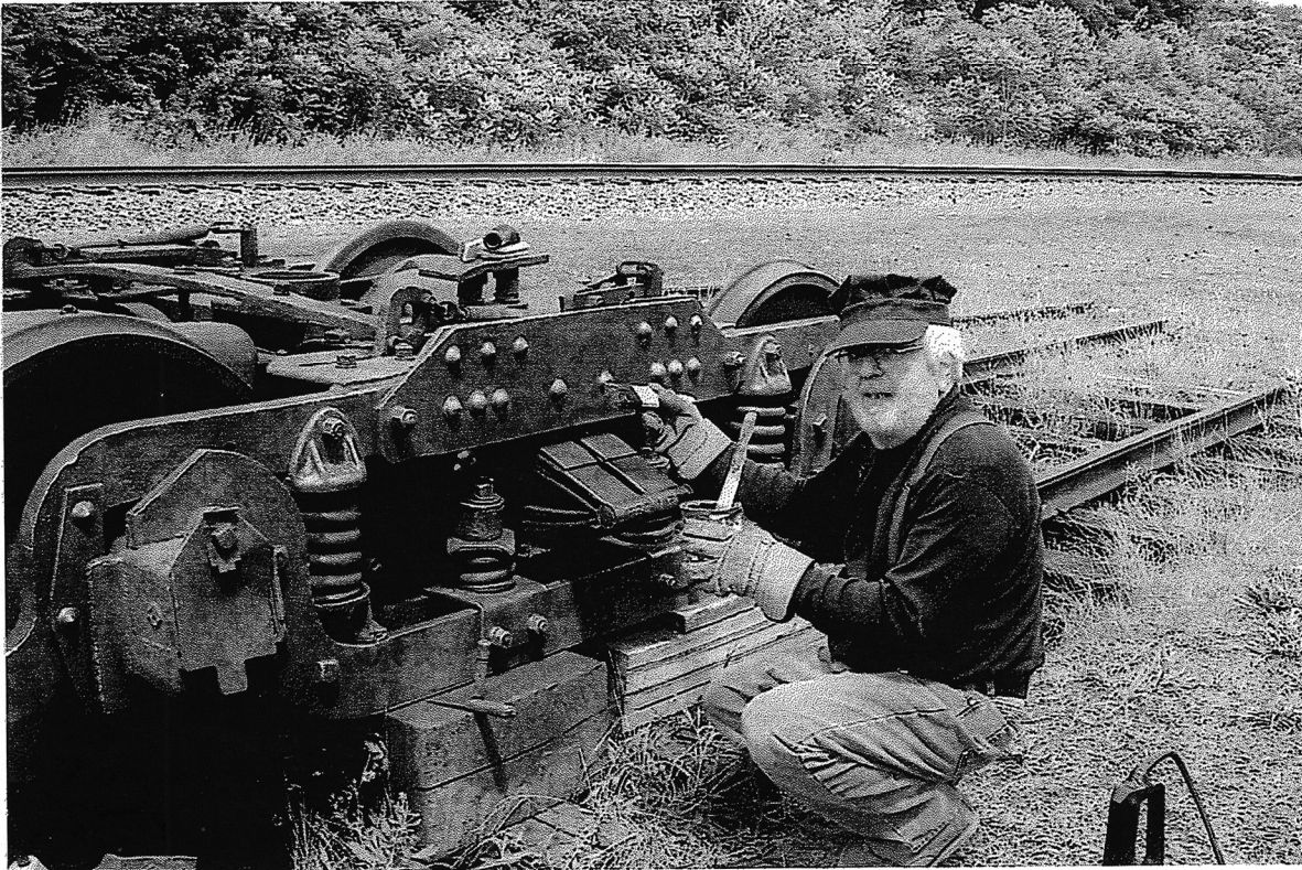
Tony Hall begins a task for which he has worked and waited for more than 35 years! Yes, cleaning and priming our ex-Boston C-60-P trucks. Bob Hooper has predicted that the trucks will have been tested and installed under the car by year's end. Photo by Bob Hooper
